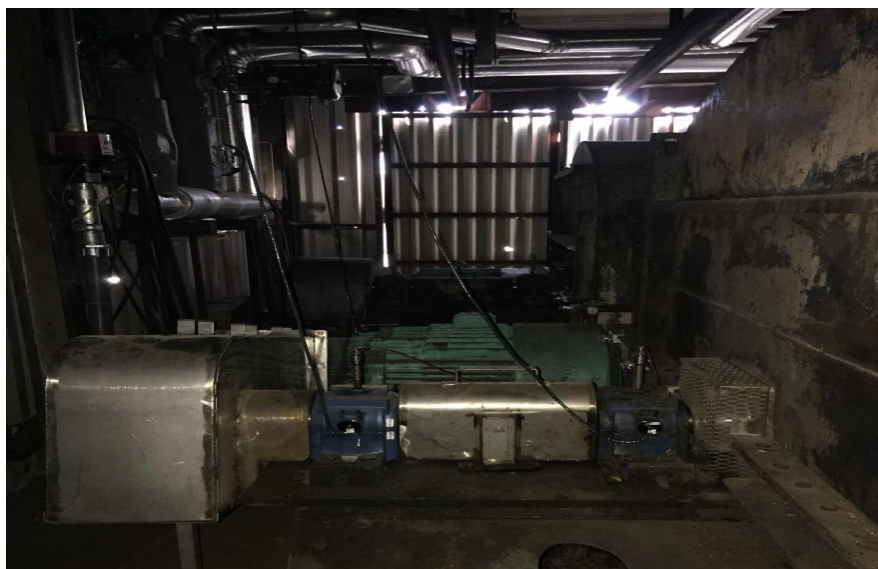
Figure 1: Exhaust fans located in a utility room on the roof where conditions included 70° C temperatures in the summer and snow and ice in the winter
