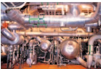
Optimum energy efficiency, e.g. in complex pumping applications
